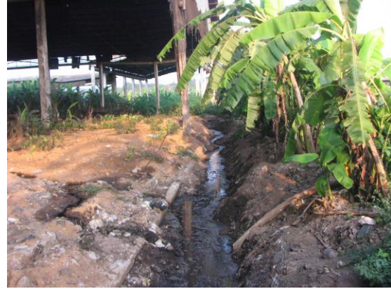
Fig. 8: Damaged drains, plantation done inside the shed area too.
