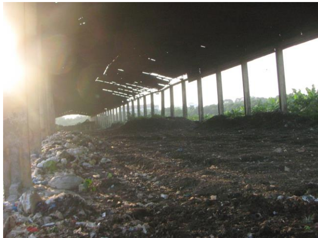
Fig.3 : Shed used for MSW storage
