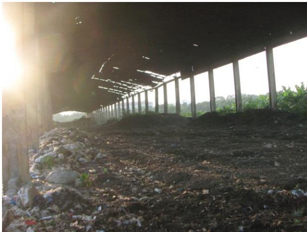
Fig.3 : Shed used for MSW storage
