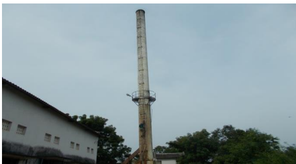
Fig 7: View of stack connected to incinerator
