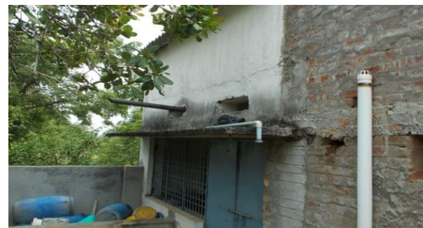
Fig 8: View of D.G.Set room where stack of D.G.Set projected side ways
