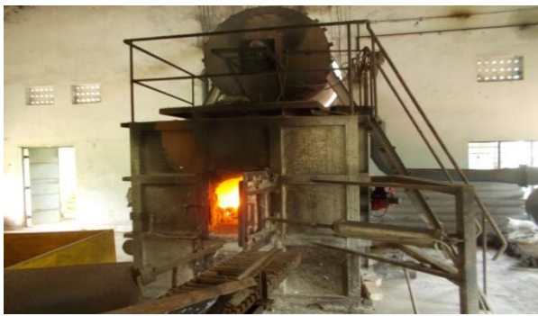
Fig 3: View of incinerator
