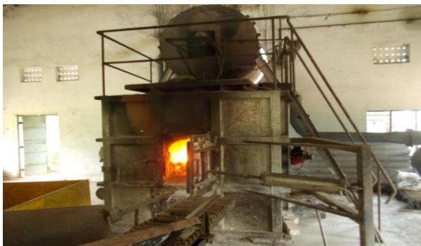
Fig 3: View of incinerator
