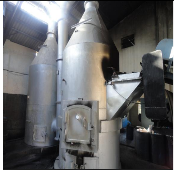
Fig.8: Primary & secondary chambers
