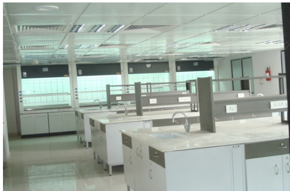
Epoxy coated ,acid & alkali proof, laboratory Tables
