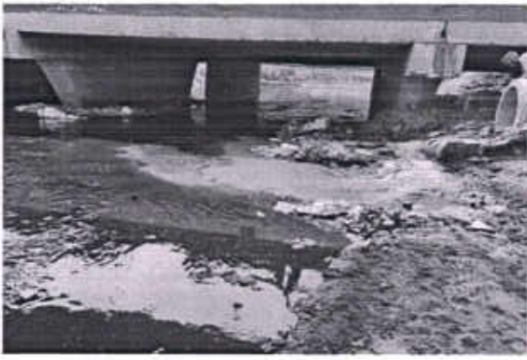
Untreated Sewage is Tibba road discharged into Budda Nallah Ludhiana directly
