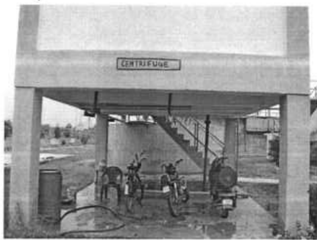
Sludge system of Jagraon East Treatment Plant is not working.(12 MLD)
