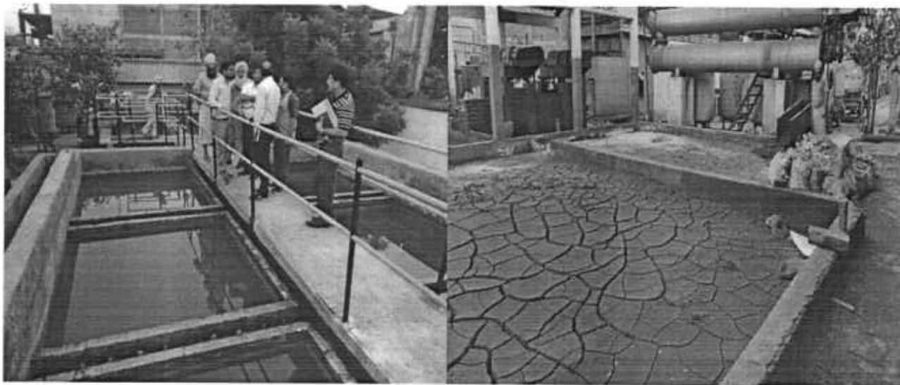
Settling Tanks for settling of solids
