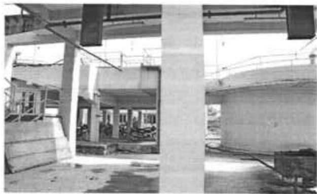
Sludge system of Hadiabad treatment plant is not working
