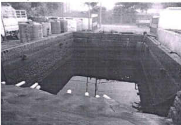
O & G Removal Tank
