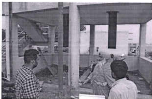
Sludge system of newly built Treatment Plant at Nakodar Jalandhar is not working
