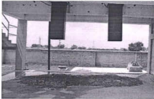
Sludge system of treatment plant of Talwandi Bhai is not working
