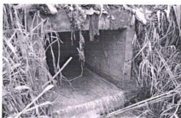
Dirty water being thrown direct into Nasrala Choe
