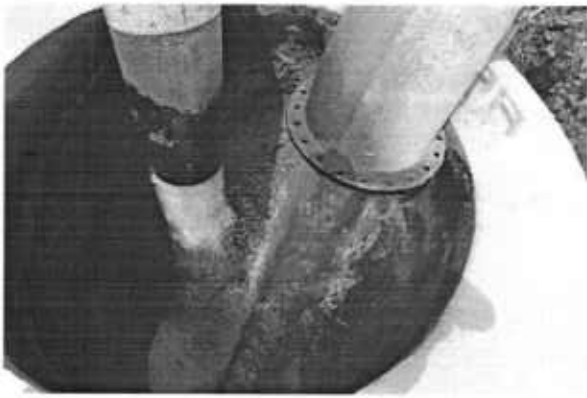
Dirty water being by passed into phagwara drain from M.P.S of Hadiabad treatment plant
