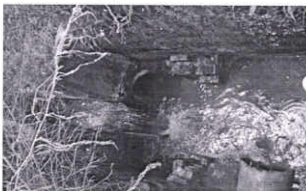
bye pass pipes of untreated water of Treatment Plant of Phillaur Jalandhar
