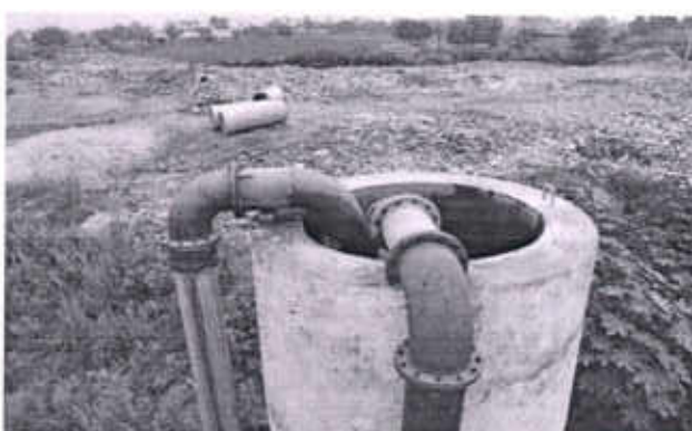
Contaminated water being thrown by pass into white Bein from Nakodar S.T.P Jalandhar
