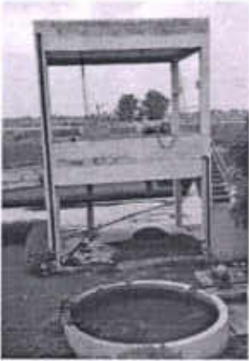
Sludge system of Zira treatment plant is not working
