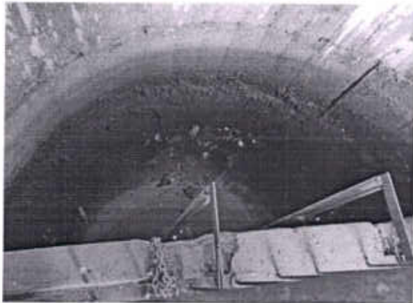
Sludge system of Rasoolpur Treatment Plant Ropar is not working
