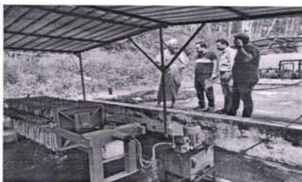
Sludge press at Brari Nangal treatment Plant is not working
