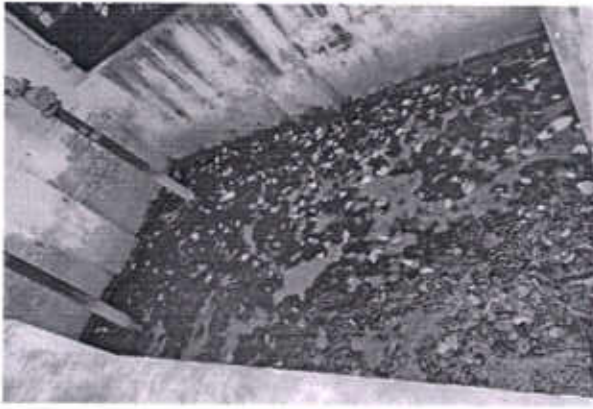
Pump system of Treatment Plant at Nangal road Ropar is not working from long time ago.
