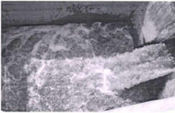
Dirty water being bye passed into the drain from Banga Treatment Plant
