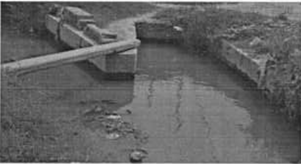
Dirty water bye passing from Kapurthala STP
