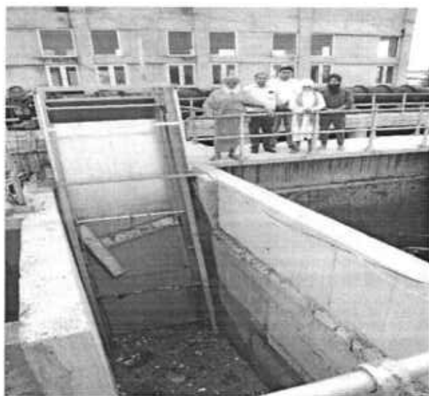
M.P.S of Basti Pirdaad Treatment Plant screen system is out of order from long time ago.
