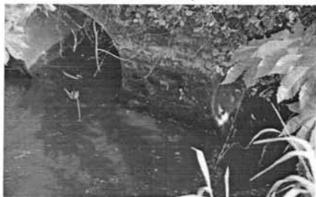
Pipes conveying untreated water to Phagwara Drain
