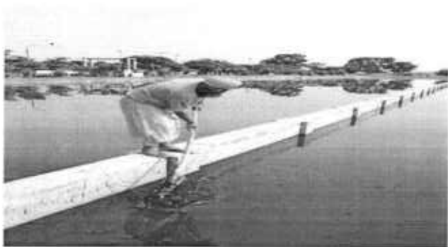
Ponds of 30 M.L.D Phagwara STP are full of Sludge
