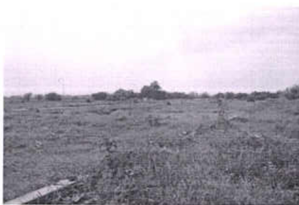
Dried up beds of 111 M.L.D Treatment Plant at Pholriwal Jalandhar which were meant for disposing off sludge
