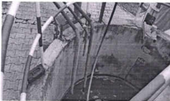
Sludge system of treatment plant at Anandpur Sahib Ropar is not operating
