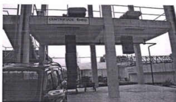
Sludge system of Mukerian treatment Plant is not working
