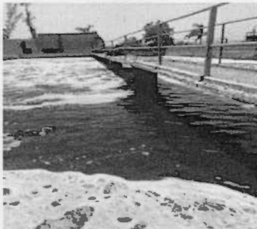
Plate-1: Photograph showing dead pocket in the aeration tank
