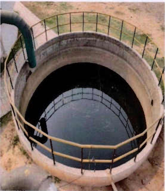
Plate-7: Final effluent collection tank
