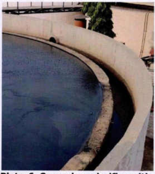
Plate-6: Secondary clarifier with dry weir
