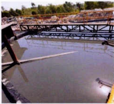
Plate-9: Primary clarifier-1
