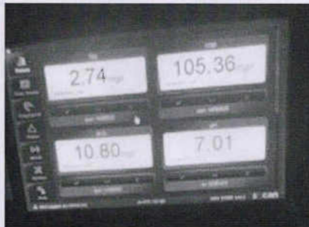
Plate-3: "Online Continuous Effluent Monitoring System" (OCEMS) showing the values of the parameters namely TSS, COD, BOD and pH.
