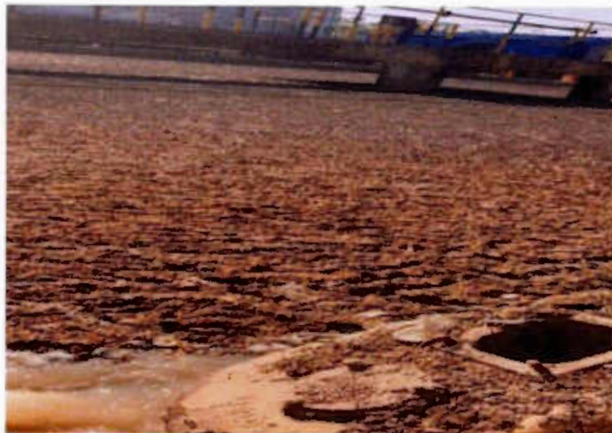
Plate-1 : Lot of scum in the equalization tank
