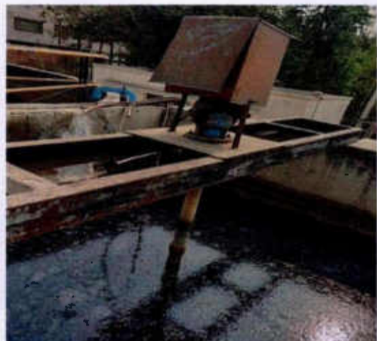
Plate-2: Flash Mixer for Chemical dosing
