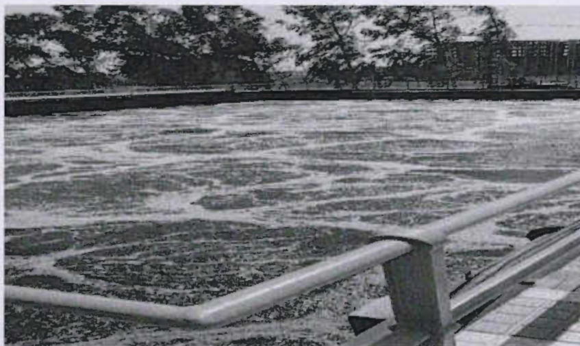
Plate-2: Effluent in aeration chamber black in colour
